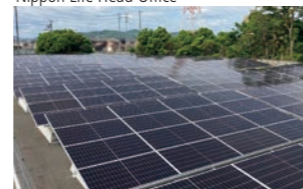
Off-site corporate PPA (Himeji City, Hyogo Prefecture)
