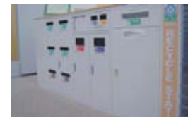
Recycle station (Tokyo headquarters)
